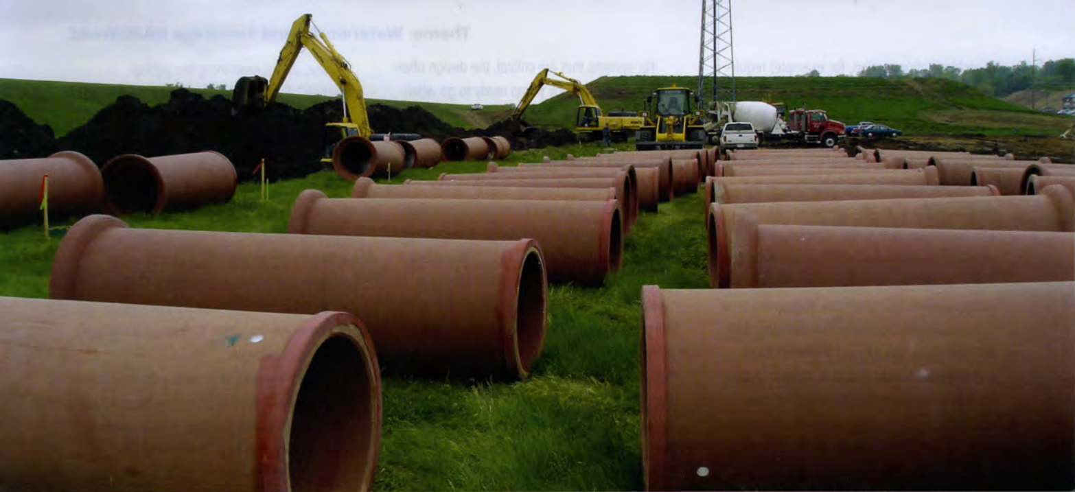
Above: 36-inch Bell and Spigot VCP (10 ft. joints), Sioux City, IA
